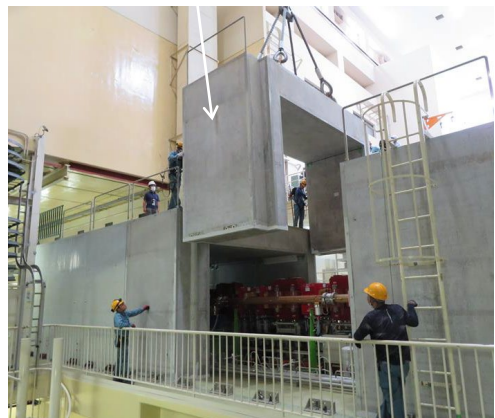
Concrete radiation shield
