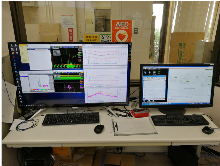
Figure 12.81: Monitoring and remote control panel by windows.
