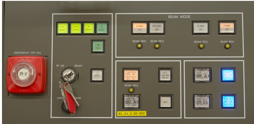
Figure 12.100: Image of the latest control panel. The beam key is used to switch the safety status from OFF, RF OK and Linac READY.
