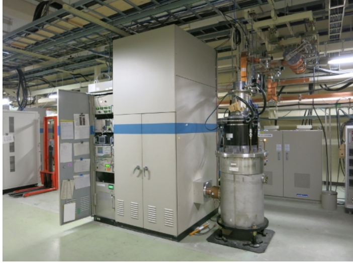
Figure 12.23: Overall view of the compact modulator with the klystron assembly and the SLED cavity.
