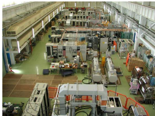
Figure 1 Klystrons, waveguide systems and control cabinets in 324-MHz klystron gallery in KEK.
