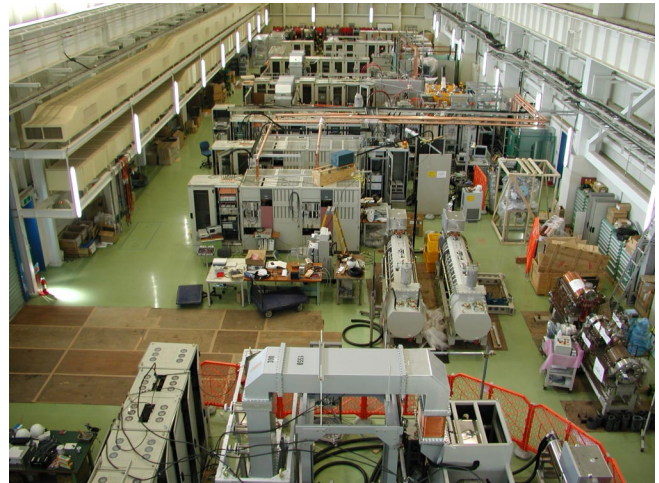
Figure 7: Klystron gallery viewed from the upstream.
