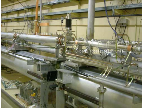
Figure 16: Photograph of the C-band acceleration unit installed in the beam-line.
