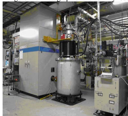
Figure 15: Photograph of the C-band unit installed in the klystron gallery.
