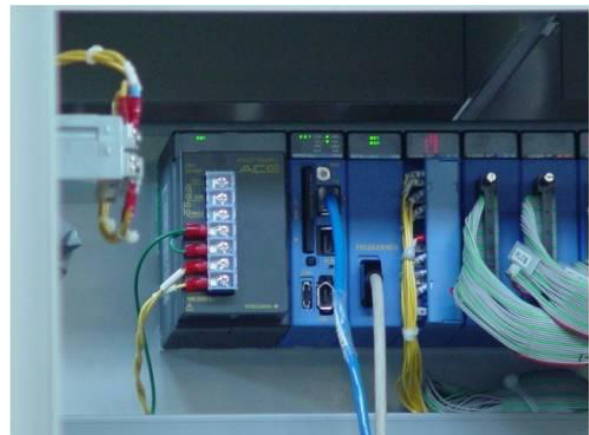
Figure 2: F3RP61 in operation.
