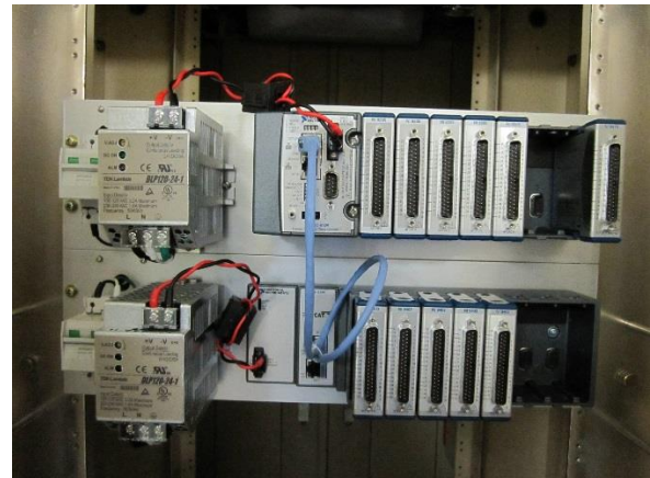
Figure 6: cRIO under installation. The light blue cable is for EtherCAT that connects main unit (upper) and extension unit (lower).
