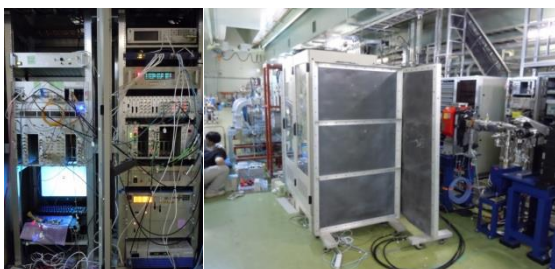
Figure 4: LLRF system for Capture Cryomodule configured inside STF Accelerator tunnel.
