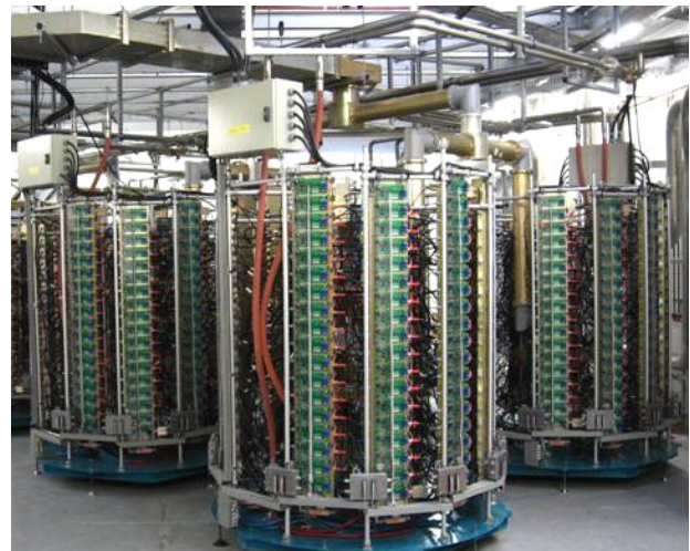
Figure 2: 180 kW SSA of the SOLEIL Storage Ring.
