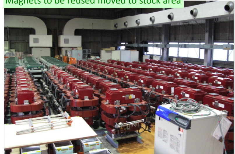
Magnets to be reused moved to stock area
