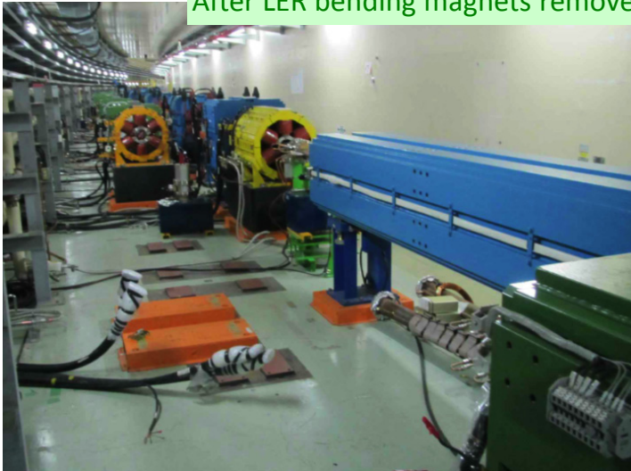
After LER bending magnets removed
