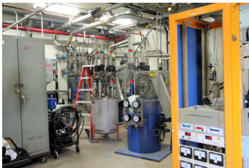
Figure 3: MTA refrigerator room.
