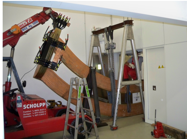
Figure 1: Bringing-in procedure of the 90° gantry dipole spare coil into the gantry hall by a specialised company.
