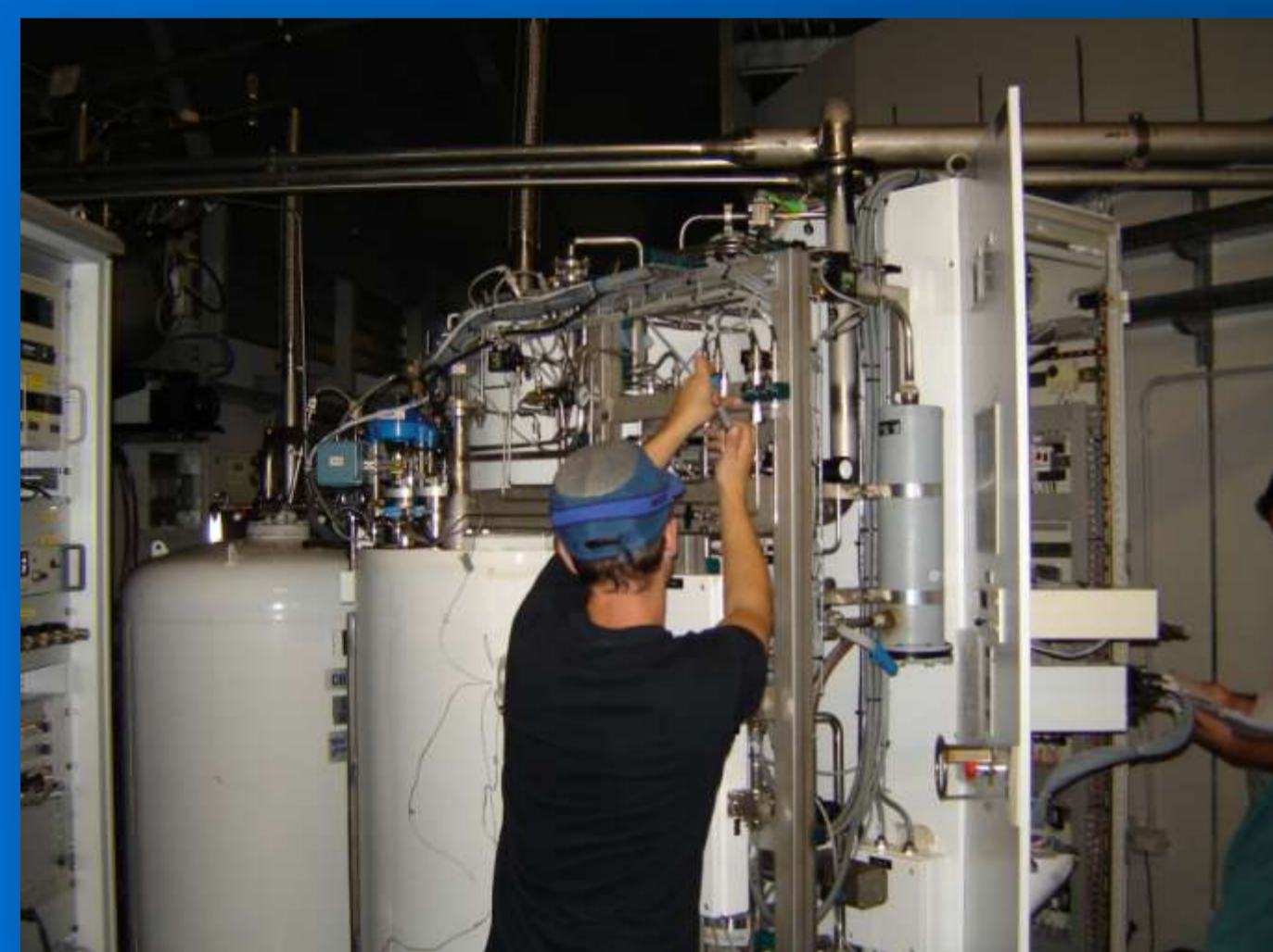
Air Liquide technician on Helial 1000 during the maintenance
