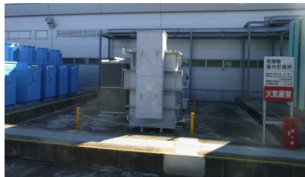
Figure 9: Storage location of the transformer-rectifier unit.
