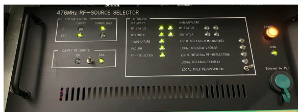
Figure 5: Photo of the RF source selector.
