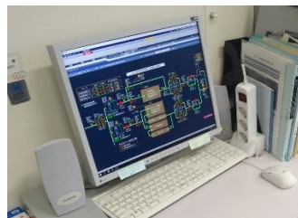
Figure 2: Proprietary workstation in the control room.
