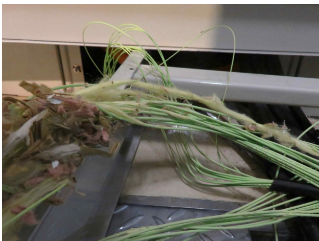
Figure 2: Damaged optical fibre cable. The outer sheath is missing and the reinforcing element is fraying.
