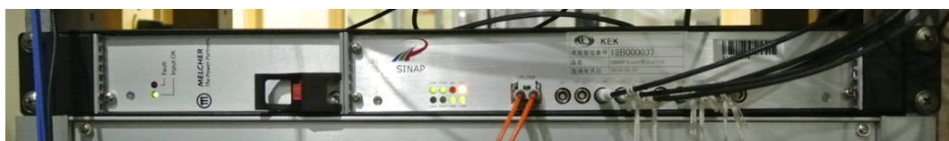
Figure 13.8: Picture of standalone EVR installed at D7: the CPU, EVR, and ethernet port are housed in the 1U height rack. The 12 timing-triggers for the LER injection are provided from this module. The triggers are provided also from rear panel. The same module is installed also at D8 and provides the timing-triggers for the HER injection.
