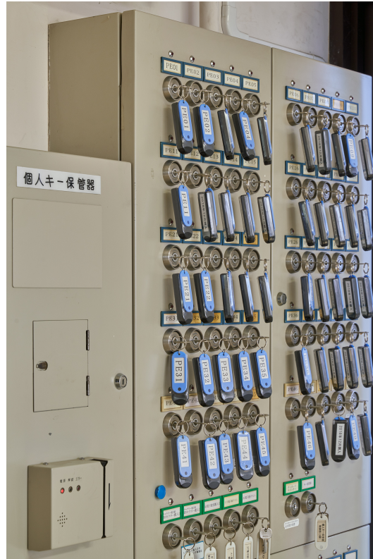
Figure 11.101: Personal keys used for entrance to the linac tunnel and the key bank.
