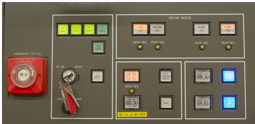
Figure 11.100: Image of the latest control panel. The beam key is used to switch the safety status from OFF, RF OK and Linac READY.
