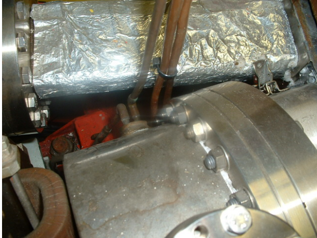
Figure 4: Elbow Water Leak
