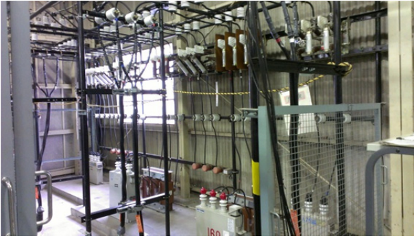
Figure 10: Newly built automatic power factor regulator.
