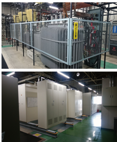
Figure 3: Transformers and switchboards before (upper picture) and after the replacement (lower).
