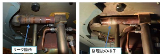
Figure 1: Location of the water leak on the cooling pipe at the klystron installed to D11-C.
