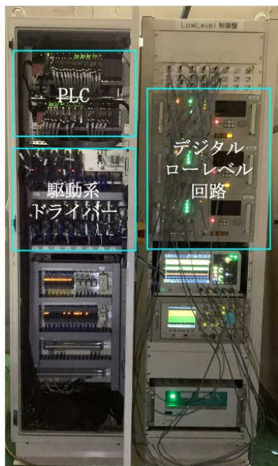
Figure 4: Low-level panel (right side of the photo) and control panel (left side of the photo) of the upgraded RF control system for RILAC injector.
