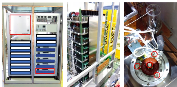
Figure 4: Interior. From left, (a) Charger and control unit. (b) MARX stack. (c) Klystron socket in Oil tank.
