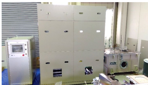
Figure 3: Exterior of modulator. From left, Control rack, High voltage stand(HVS), Oil tank.
